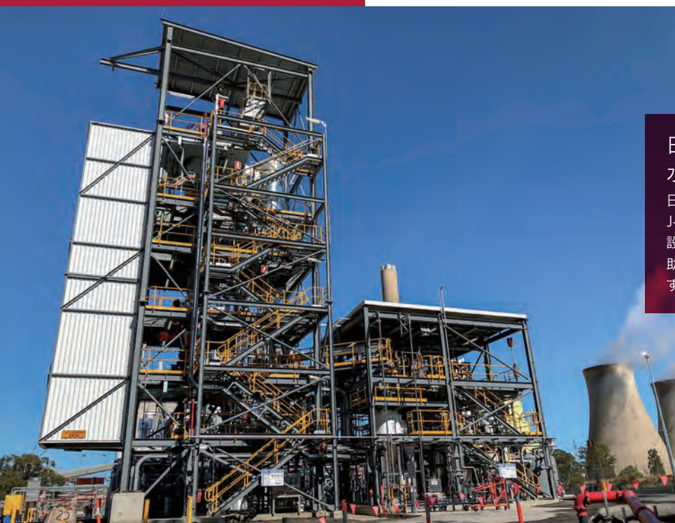
写真提供：HySTRA, J-POWER / J-POWER Latrobe Valley
