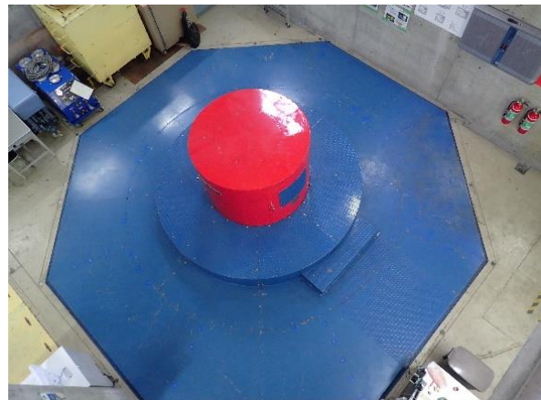
Inside the power station (power generation equipment)
