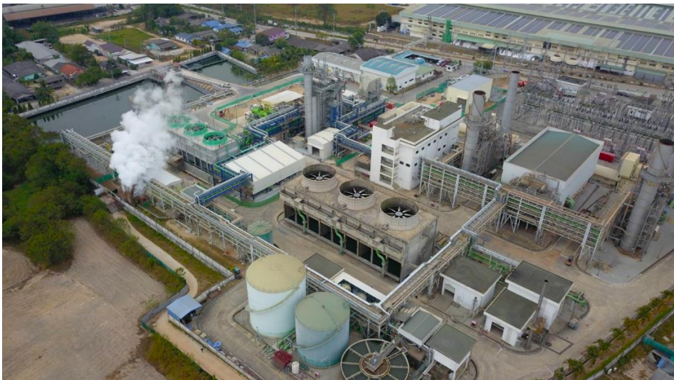
EGCO Cogen Gas Cogeneration Power Plant
