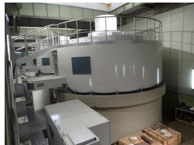
Inside (power generation equipment)
