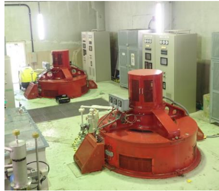
Inside (power generation equipment)
