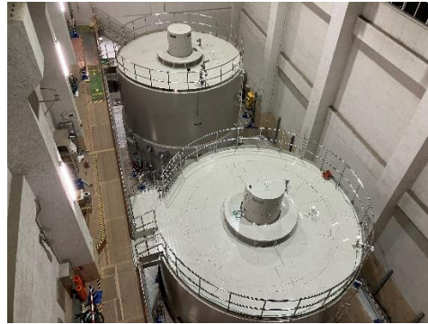
Inside the power plant (front: Unit 1, back: Unit 2)
