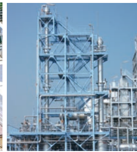
CO 2 separation and recovery facility
