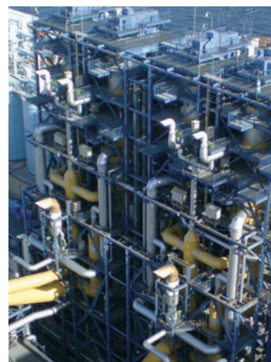
Dry-type desulfurization system at Isogo New No. 2 Thermal Power Plant
