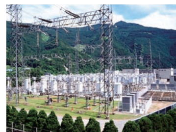
Sakuma Frequency Converter Station (Shizuoka Prefecture)
