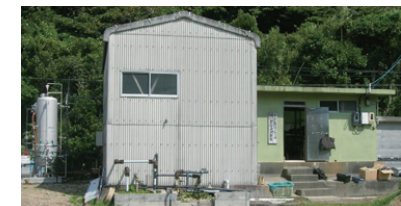
Decentralized water supply (Ishima small-scale water supply)
