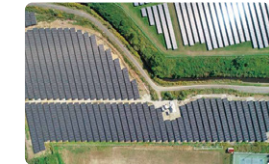
Himeji Oshio Solar Power Plant, Hyogo Pref. Owned capacity: 1.999 MW
