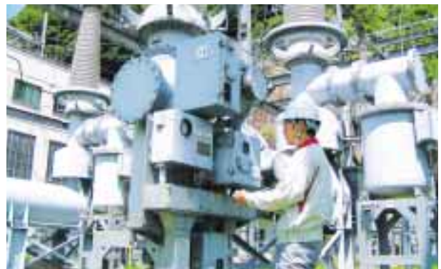
Inspection of gas pressure of switches (Sakuma Power Station)
