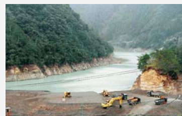
Responding to sediment (Futatsuno Regulating Reservoir, Nara Prefecture)
