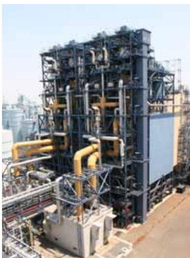
Dry-type desulfurization system at Isogo Thermal Power Station new No. 2 unit (Yokohama)
