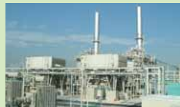
Ichihara Power Station (Bay Side Energy Co., Ltd., Chiba Prefecture)
