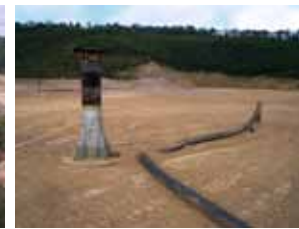
Landfill gas *3 recovery well
