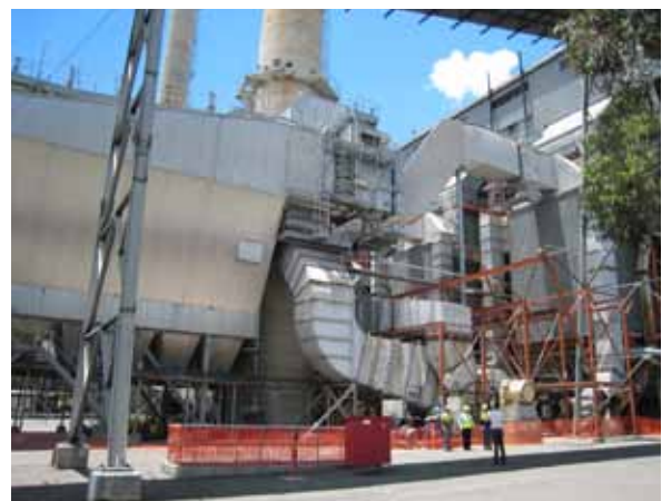
Callide Coal-fired Thermal Power Station (Australia)
