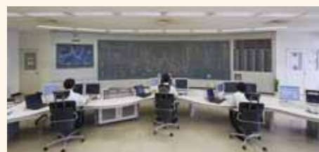
Central Load Dispatching Center
