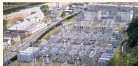
Sakuma Frequency Converter Station (Hamamatsu)
