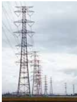
Tadami Main Transmission Line (Gunma Prefecture)
