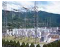
Sakuma Frequency Converter Station
