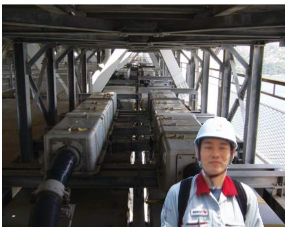
500,000-volt transmission cable installed on Seto Ohashi Bridge
