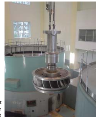
Total upgrade of main equipment at Nukabira Power Station (Hokkaido)
