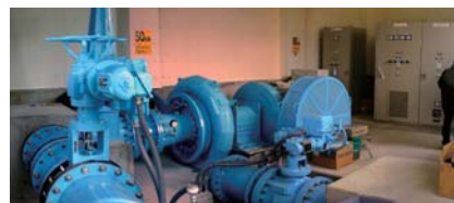
Yokkaichi Bureau of Waterworks hydroelectric power station (Mie Prefecture, 320 kW), for which KDC Engineering Co., Ltd. provided design and construction supervision.
