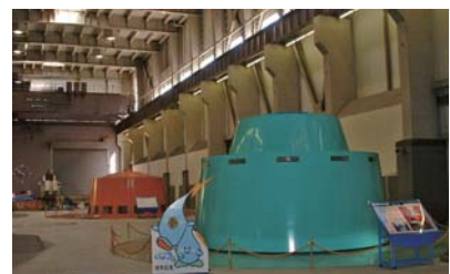
Okukiyotsu No. 2 Power Station (Variable-speed pumped-storage generating system)
