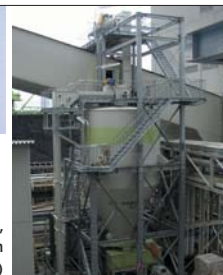
Biosolid supply facility, Matsuura Thermal Power Station (Nagasaki Prefecture)
