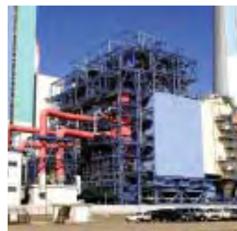
Dry-type flue-gas desulfurization system at Isogo Thermal Power Station's new No. 1 unit.
