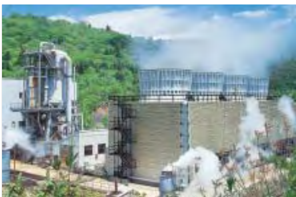
Onikobe Geothermal Power Station (Miyagi Prefecture)
