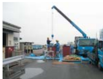
Machinery containing PCBs being shipped to treatment site (Wakamatsu Operations & General Management Office, Fukuoka Prefecture)
