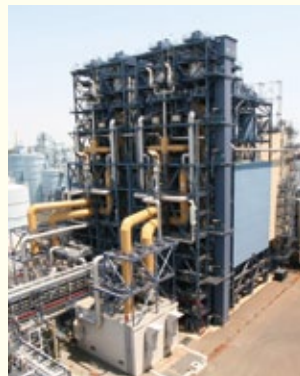
Dry desulfurization unit (Isogo Thermal Power Station, new Unit 2)
