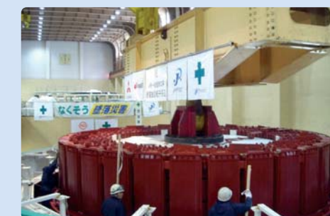
Tagokura Power Plant Comprehensive renewal of main electrical equipment
