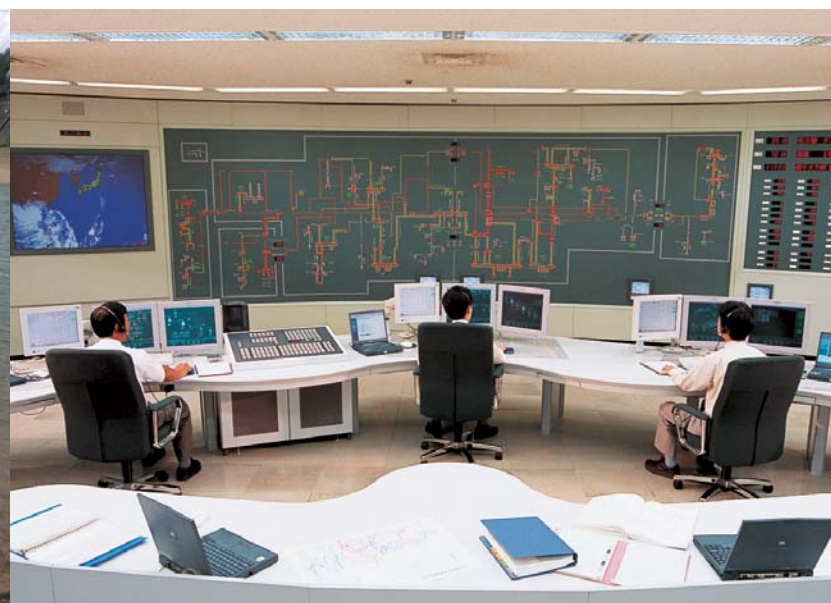
Central Load Dispatching Center
