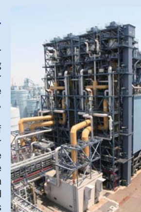
Dry Type Desulfurization System (New No.2 Unit of Isogo Thermal Power Plant)
