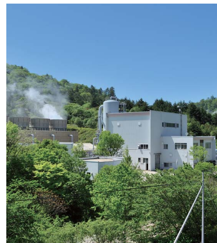
Onikobe Geothermal Power Plant
