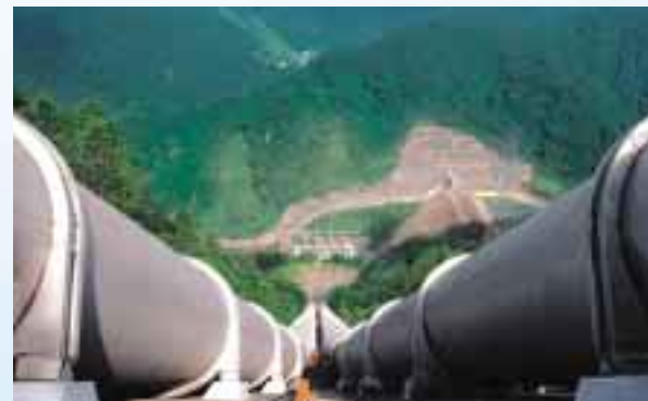
Okukiyotsu Power Plant
