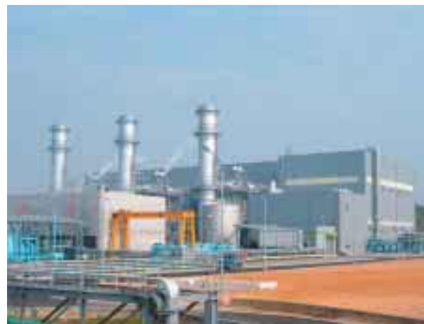
Chiahui Gas Combined Cycle Power Plant ( Taiwan ) [ IPP ]
