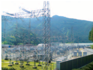
Sakuma Frequency Converter Station (Shizuoka Prefecture)
