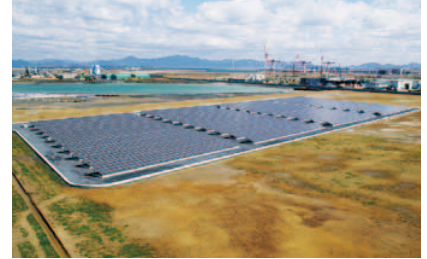
Hibikinada Solar Power Station (Kitakyushu City)
