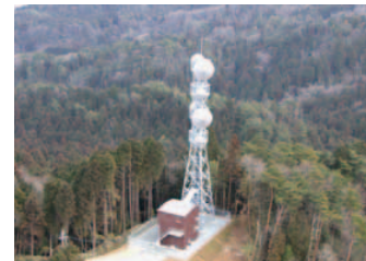
Tsuge Radio Relay Station (Nara Prefecture) A microwave radio relay station that links power stations, transformer stations, and other facilities. The station is highly reliable in order to ensure uninterrupted communications even in the event of a disaster such as an earthquake or typhoon.
