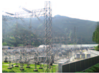
Sakuma Frequency Converter Station (Shizuoka Prefecture) This converter station enables the transmission of electricity between the different frequencies of eastern Japan (50 Hz) and western Japan (60 Hz). It is the world's first electricity business frequency converter station built to support efficient electric power operations.
