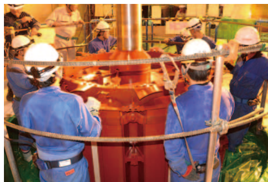
A view of the generator (rotator) suspended (Isawa Hydroelectric Power Station, Iwate Prefecture)
