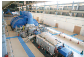
The turbine generator in the Isogo Thermal Power Station
