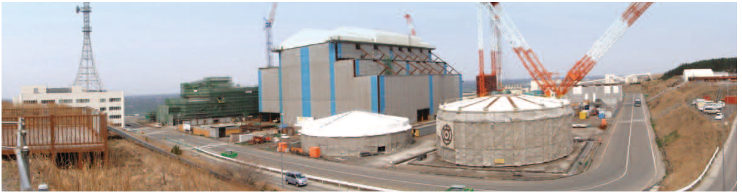
Panoramic view of construction work on Ohma Nuclear Power Station (Aomori Prefecture)
