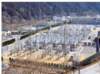
Sakuma Frequency Converter Station (Shizuoka Prefecture)
