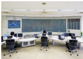
Central Load Dispatching Center
