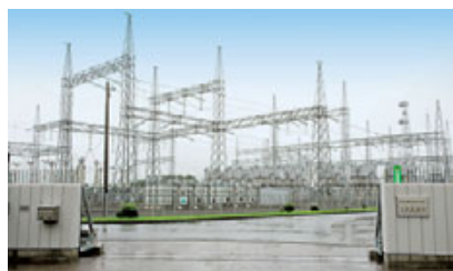
Kitahon HVDC Link Kamiyama Converter Station (Aomori Prefecture)
