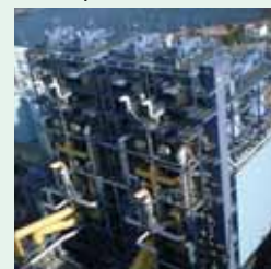
Dry-type desulfurization system at Isogo Thermal Power Station new No. 2 unit (Yokohama)
