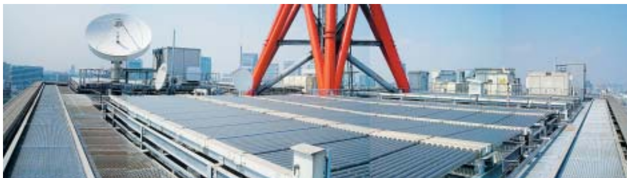
Solar panels for the indoor hot-water supply system in J-POWER headquarters (roof of head office building, Tokyo)
