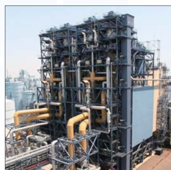
Dry type desulfurization plant
