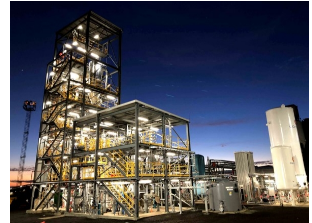
Brown coal gasification facility Source: HySTRA
