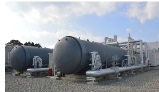
Fuel cell modules Solid Oxide Fuel Cell (SOFC) Capacity : 1.2MW class (0.6MW class SOFC X2)
