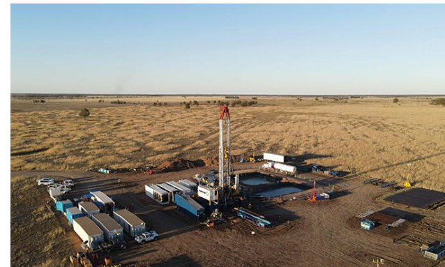
CO 2 injection site near Moonie in Queensland, Australia
