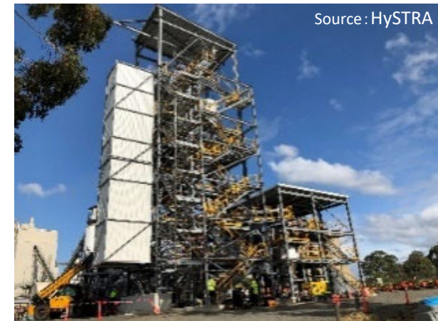
Brown coal gasification facility
