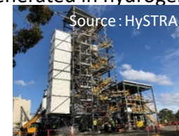
Brown coal gasification facility
