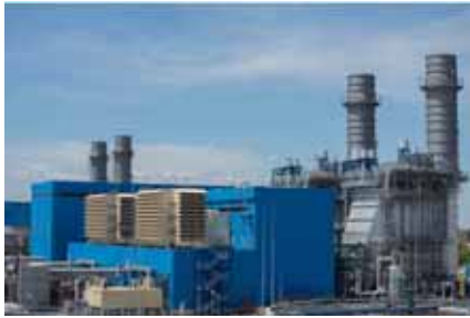
NS IPP (2014, in operation)
