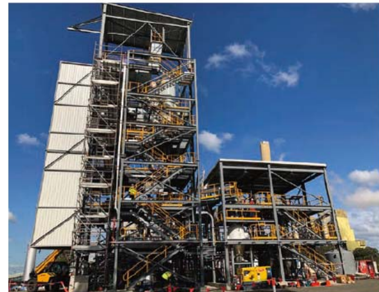
A brown coal gasification furnace and hydrogen production test equipment being constructed in Australia (Photo courtesy of HySTRA)
