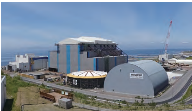
Construction status of the Ohma Nuclear Power Plant Project (as of June 2019)
