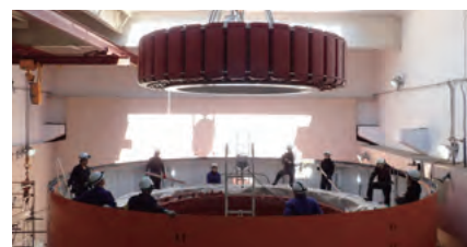
Akiba No. 1 Repowering (Shizuoka Prefecture)
