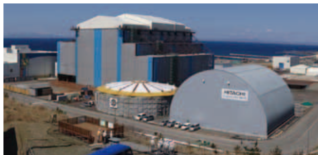
Construction status of the Ohma Nuclear Power Plant Project (as of June 2018)
