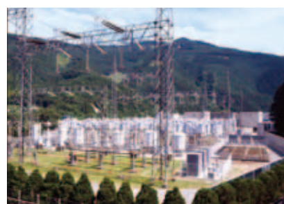
Sakuma Frequency Converter Station
