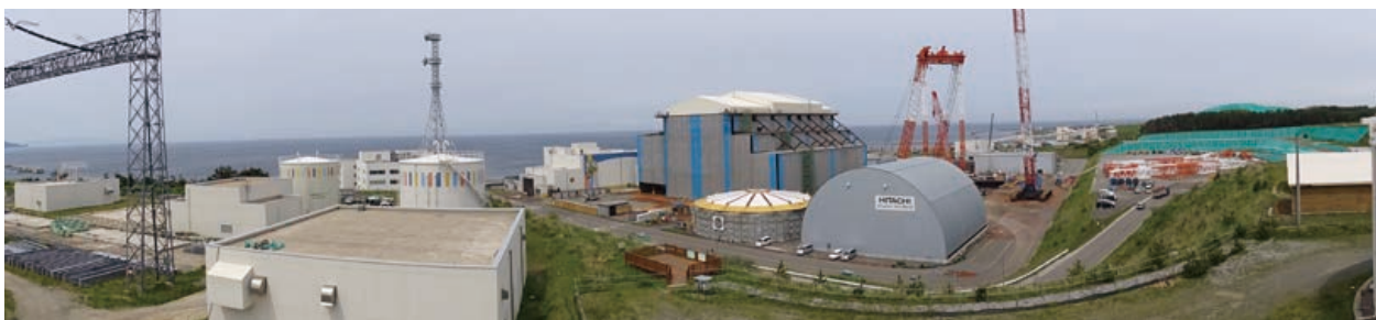
Construction status of the Ohma Nuclear Power Plant Project (as of June 2017)
