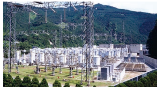
Sakuma Frequency Converter Station
