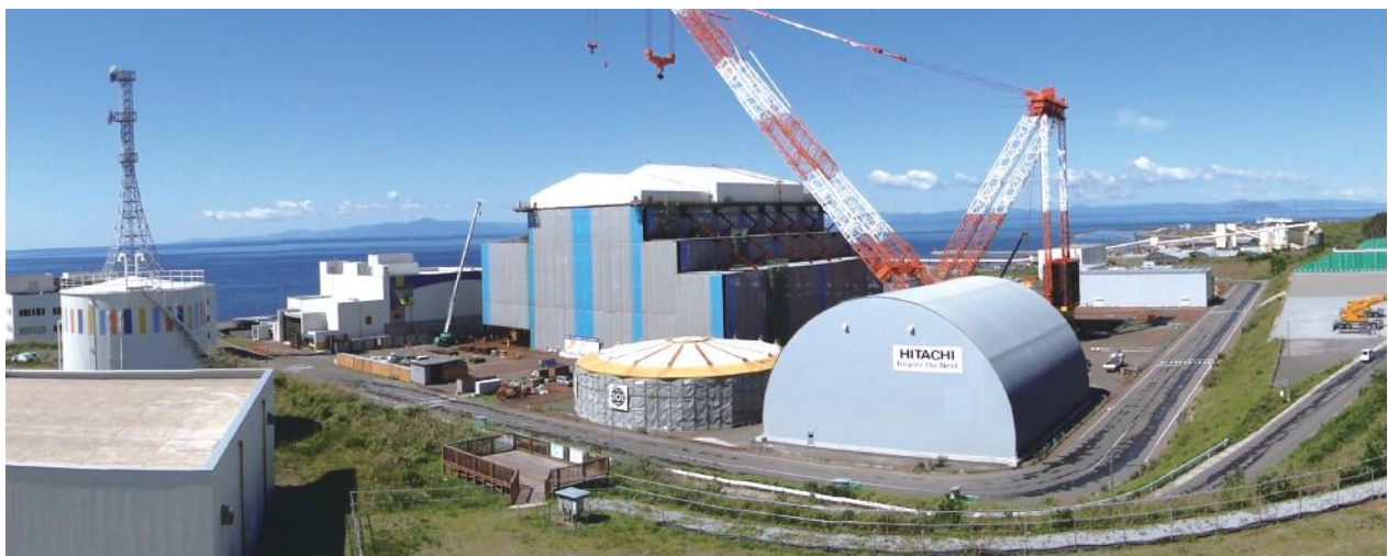
Panoramic view of construction work on Ohma Nuclear Power Plant (Aomori Prefecture)
