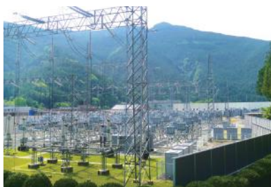
Sakuma Frequency Converter Station (Shizuoka Prefecture) This converter station enables the transmission of electricity between the different frequencies of eastern Japan (50 Hz) and western Japan (60 Hz). It is the world's first electricity business frequency converter station built to support efficient electric power operations.
