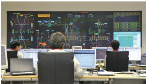
North Regional Control Center (Hokkaido)
