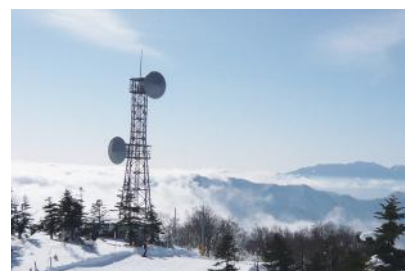
Takatsue Radio Relay Station (Fukushima Prefecture) A microwave radio relay station that links power stations, transformer stations, and other facilities. The station is located on the top of a mountain, where environmental conditions are extreme, but it is highly reliable in order to ensure uninterrupted communications even in the event of a disaster.
