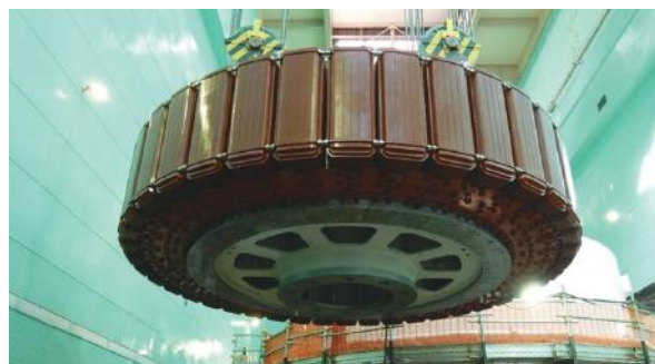
Rotor being lifted into place at Akiba No. 2 Power Station (Shizuoka Prefecture)
