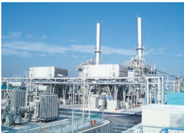
Bayside Energy Ichihara Power Plant (Chiba Prefecture)
