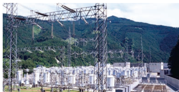
Sakuma Frequency Converter Station
