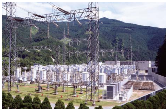
Sakuma Frequency Converter Station
