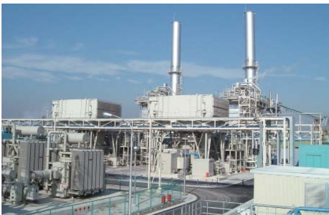
Bayside Energy Ichihara (Chiba Prefecture)
