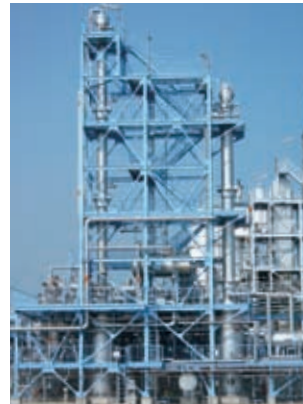
CO 2 separation and capture facility
