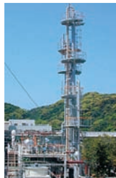
Test facilities for CO 2 separation and capture at the Matsushima Thermal Power Plant's Unit 2
