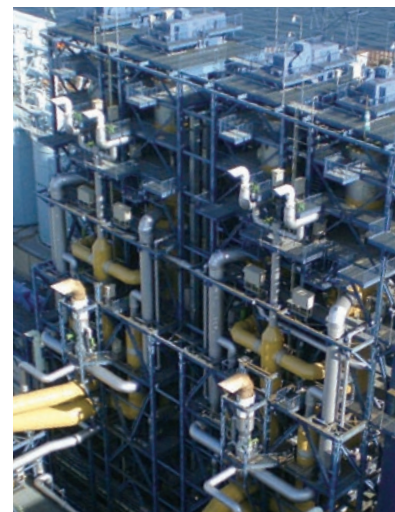
Dry-type desulfurization system at Isogo New No. 2 Thermal Power Plant
