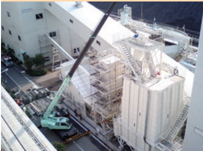
Wood biomass handling facility (Matsuura Thermal Power Plant)
