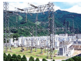
Sakuma Frequency Converter Station (Shizuoka Prefecture)
