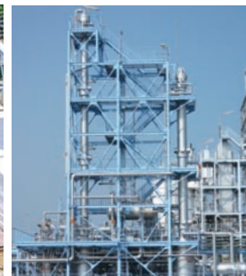
CO 2 separation and recovery facility
