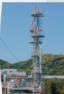
Facility for demonstrating CO 2 separation and recovery at the Matsushima Thermal Plant, Unit 2
