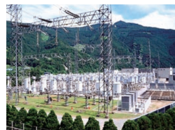
Sakuma Frequency Converter Station (Shizuoka Prefecture)
