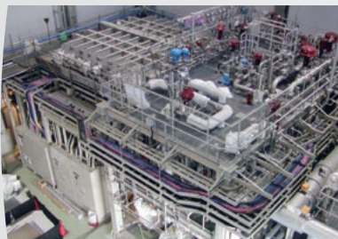
Atmospheric pressure SOFC cogeneration system (150 kW-class) (Chigasaki Research Institute)
