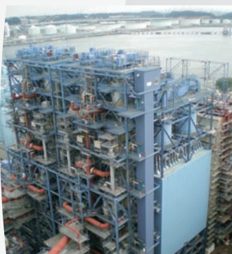
Dry-type desulfurization system at Isogo New No. 2 Thermal Power Plant
