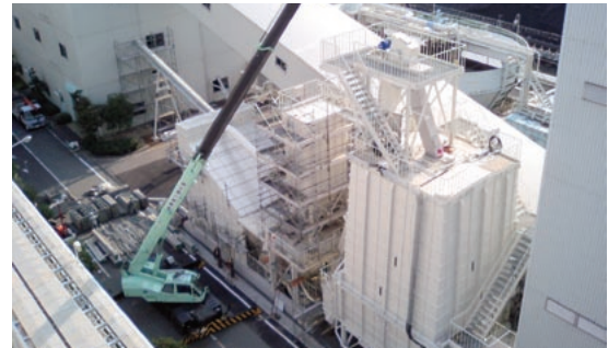
Wood biomass handling facility (Matsuura Thermal Power Plant, Nagasaki Prefecture)
